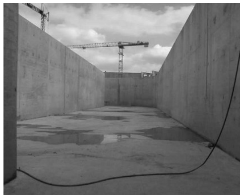
Fig. 15. The biological tank of a wastewater treatment plant
